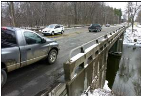
(ROD SANFORD/Lansing State Journal) Popular byway: Traffic moves Monday on Hagadorn Road over the Red Cedar River in East Lansing. Some 27,600 vehicles per day pass over this bridge, which is rated one of the most structurally deficient in the Lansing area. The bridge was built in 1930.
